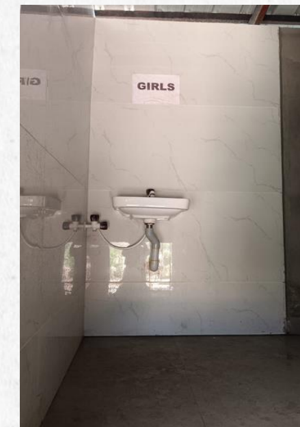
Washroom in our school Only sink; no dustbins
